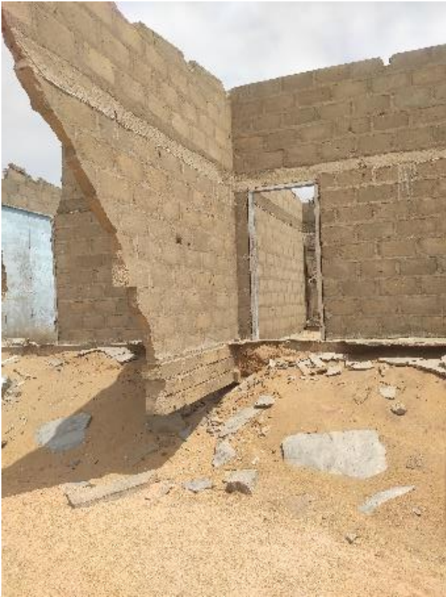
Figure 4: Affected house in Agavedzi. Source: Own photo with permission of the residents.
